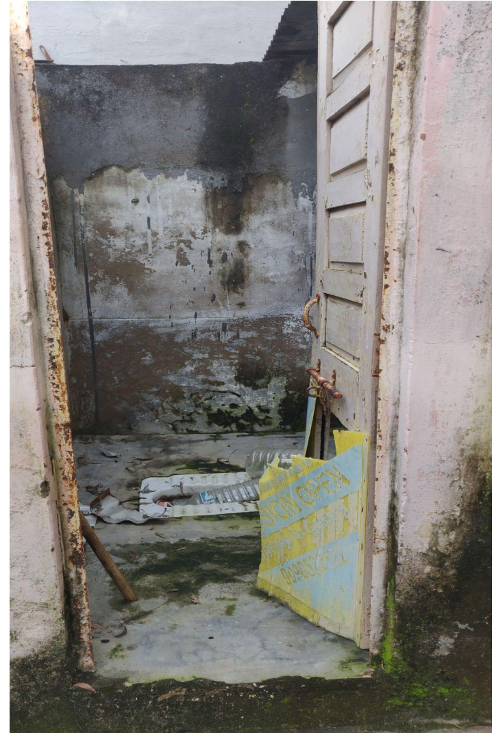
Condition of Toilet in a government school
